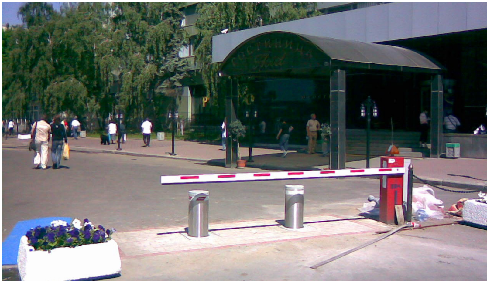
Installation with automatic rising bollards 275/P 800A
